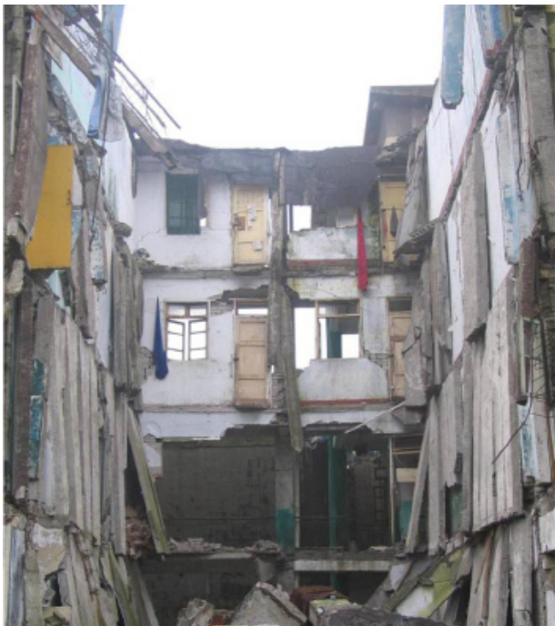
Collapse due to precast floor panels slipping off the supporting wall (May 2008 earthquake - Wenchuan, China). GHI identified a similar risk in Indian schools.
