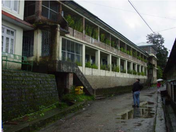
Bill Holmes assesses seismic vulnerabilities of a building in the Tibetan Children's Village in Dharamsala.
