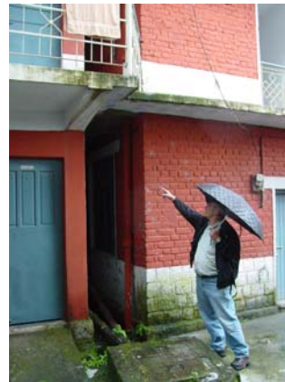
Attention is drawn to poor connections between buildings too closely built.
