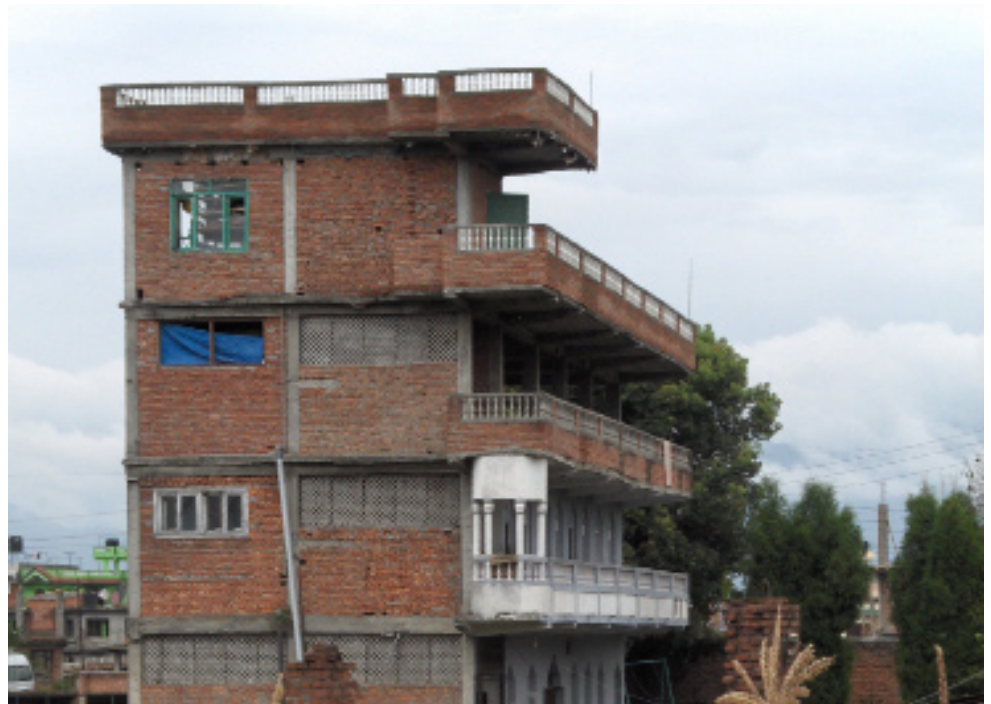
(Above) A dangerous building in Kathmandu, Nepal. The grey concrete columns and beams, which form structural “frames,” have been filled in an indiscriminate manner with red, unreinforced bricks.
